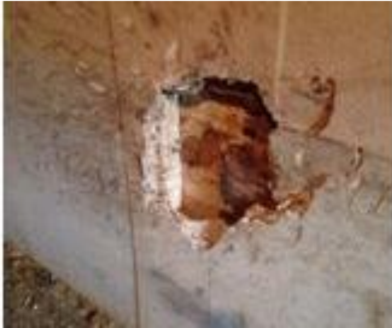
Figure 10. Damage to stable wall
