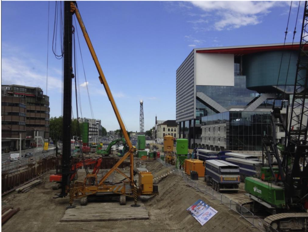
Fig. 3. Construction of pedestrian and cycling walkways for Utrecht Station Area Redevelopment (USARP) in the Netherlands. Source: Authors (2014).
